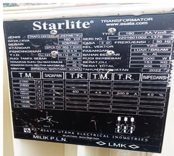
Gambar 4. Nameplate Transformator Starlite
